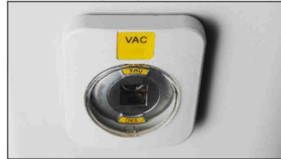
Gas outlet with shield
